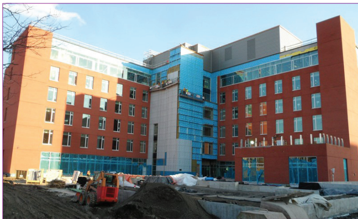
Construction continues on the new Intergenerational Wellness Centre, which will house CAMH's Geriatric Mental Health Program and Child, Youth and Family Program
